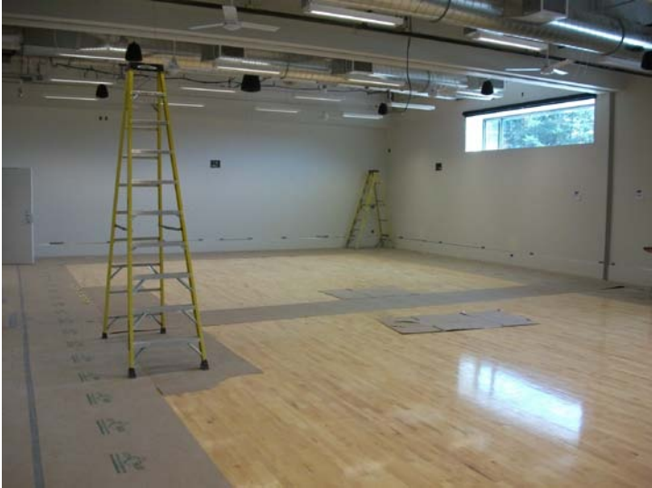
Wood flooring in Group Exercise Room
